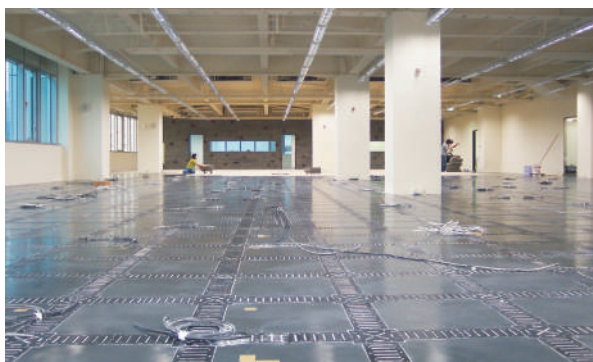
Cables routing inside the Cable Trenches and extending through any point of the interiors
